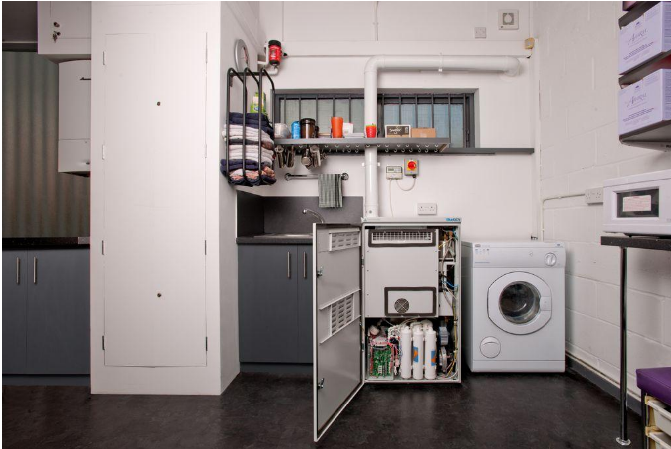
BlueGen showing access to water treatment filters
