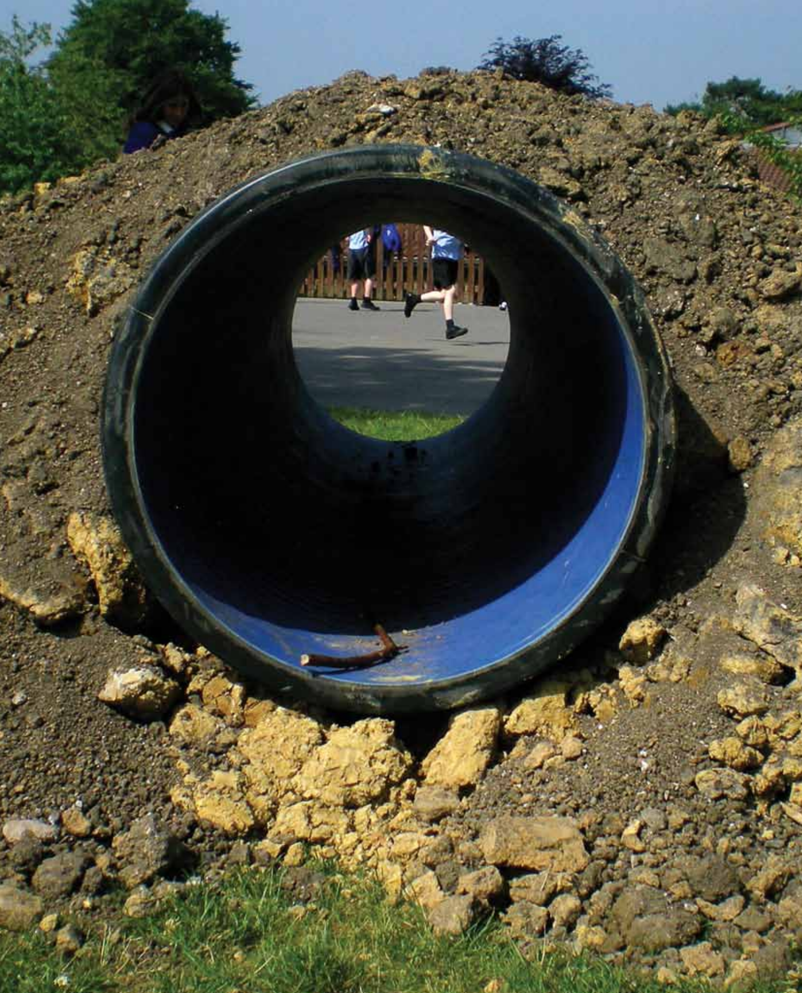
Playground improvements under construction at Manor Primary School, South Gloucestershire; designed and part-funded by the pupils themselves. A cluster of similar projects were supported locally under the 'Narrowing the Gap' programme of the National College for School Leadership. Further information: andy.grant@thecastleschool.org.uk
