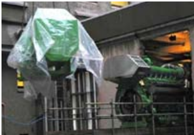
A CHP facility at the University
